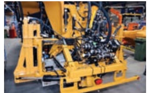
Special hydraulic hoses and piping
